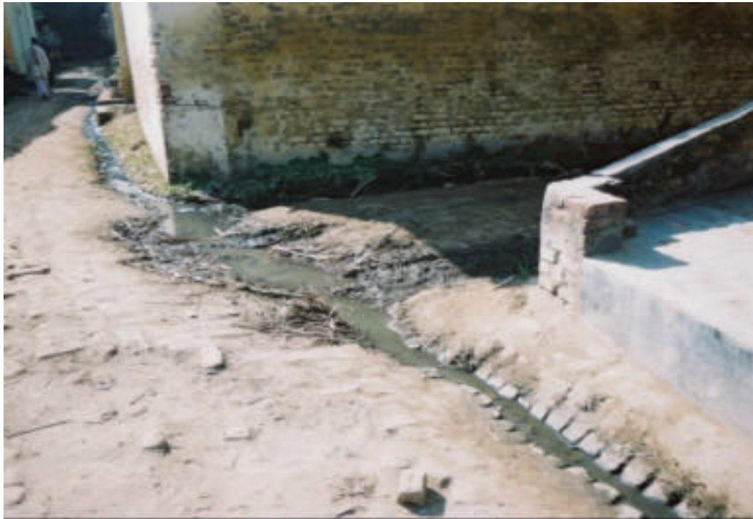
Pitiable Condition of Drainage System (Picture)
