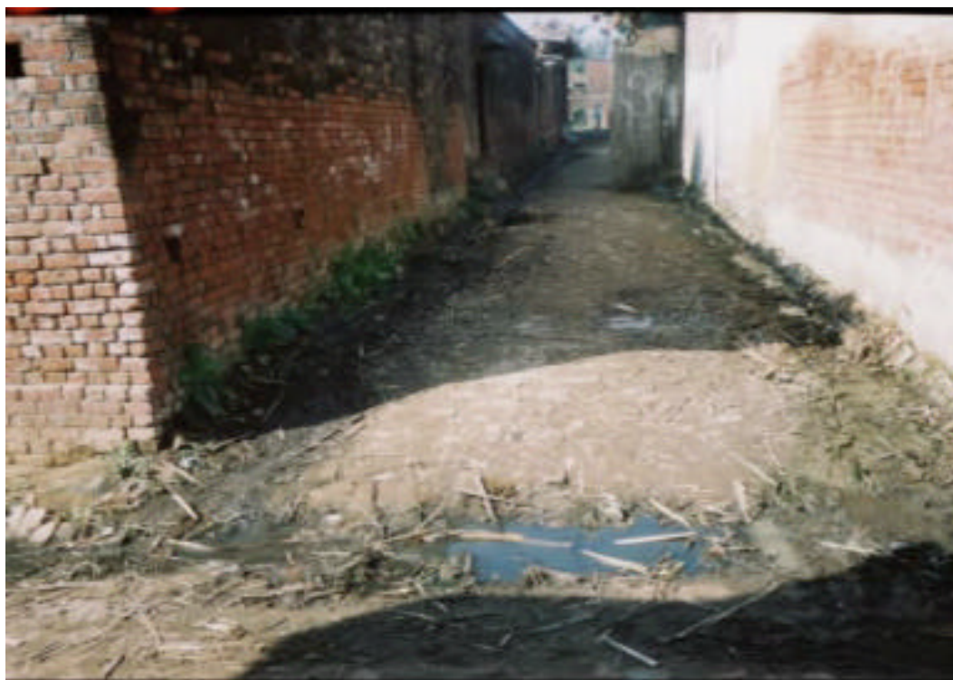
Condition of the Village Roads (Picture)
